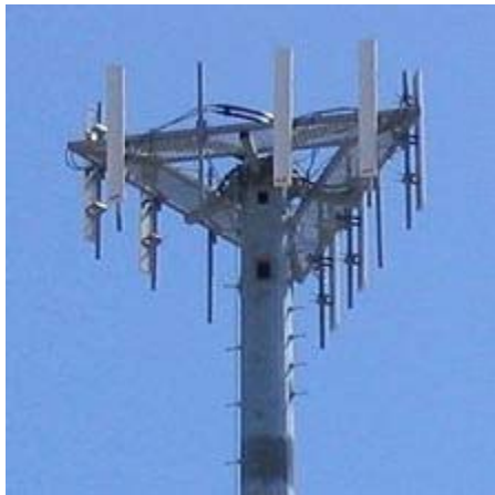
Top of cellular telephone tower
